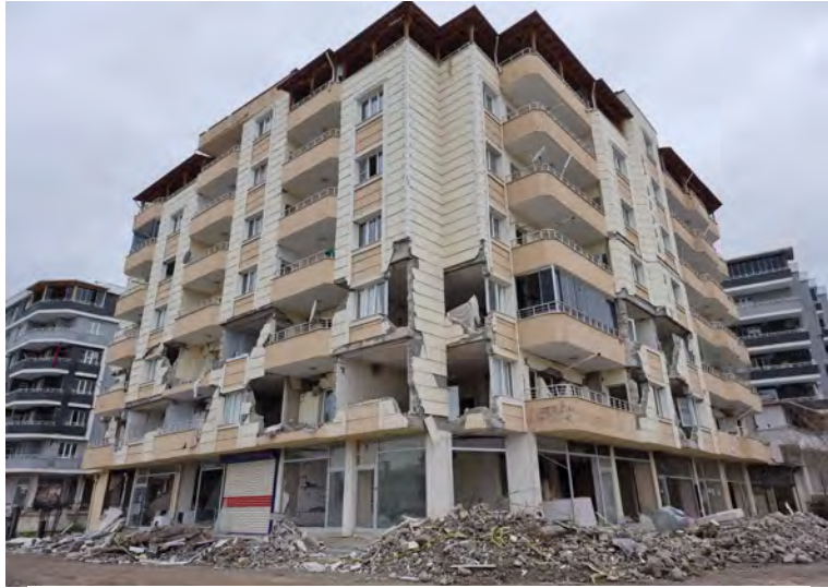
Damage after 2023 Turkey EQs
